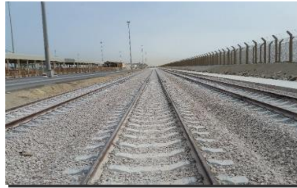
CONNECTION OF 2 nd CONTAINER TERMINAL INSIDE KING ABDUL AZIZ PORT IN DAMMAM WITH THE EXISTING RAILWAY
