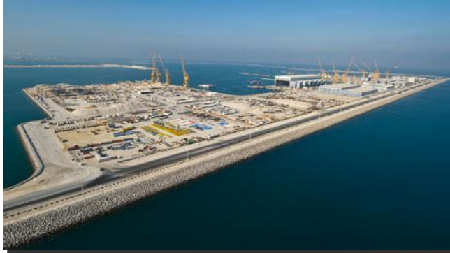
MARINE WORKS FOR (PHASE 5), ERHAMA BIN JABER AL-JARALLAH SHIPYARD, PORT OF RAS LAFFAN
