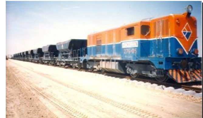
RENEWAL OF 100 KM OF TRACK BETWEEN SIDING 9 AND RIYADH AT SECTIONS H, I, AND J
