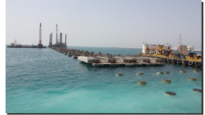
EPC OF CIVIL AND MEPI WORKS (PHASE 2A) FOR THE ERHAMA BIN JABER AL JALAHMA SHIPYARD
