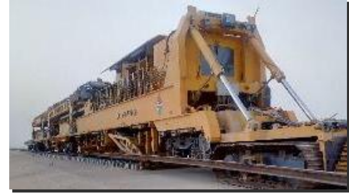
SAUDI RAILWAY PROJECT CTW-110 TRACK LAYING SCOPE FROM RAS AL KHAIR TO JUBAIL INDUSTRIAL CITY
