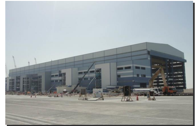
PROCUREMENT AND INSTALLATION OF M&E SERVICES, NAKILAT SHIP REPAIR YARD (PHASE 1 & 2) AND SHIP CONSTRUCTION FACILITY (PHASE 4)
