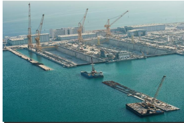
CONSTRUCTION OF CIVIL AND BUILDING WORKS, PHASES 4A & 5, NAKILAT SHIP REPAIR YARD, RAS LAFFAN
