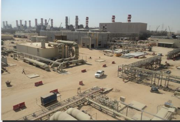
RAS AL-KHAIR POWER AND DESALINATION PLANT, JUBAIL
