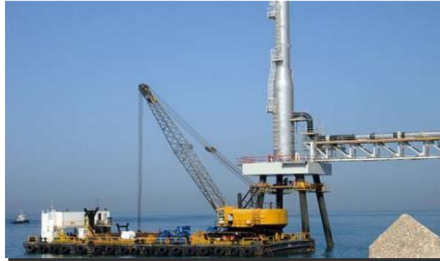
FLARE SUPPORT STRUCTURE, BERTH NO 4, QGII LNG ONSHORE FACILITIES PROJECT, RAS LAFFAN
