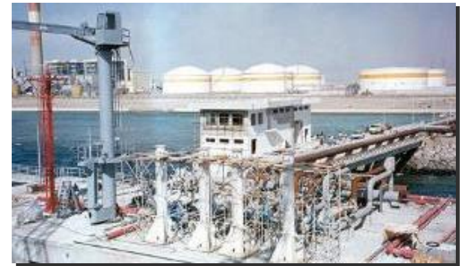
LOCAL FUEL RECEIVING TERMINAL AT RABIGH STEAM POWER PLANT
