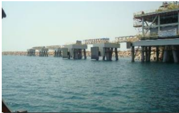
MARINE CIVIL WORKS FOR LNG BERTH NO 5, QGII LNG ONSHORE FACILITIES PROJECT, SUPPLY AND CONSTRUCTION, RAS LAFFAN
