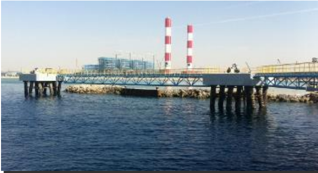
YANBU POWER PLANT (2700 MW) WORKS FOR OFFSHORE TERMINAL (JETTY WORKS), YANBU PLANT
