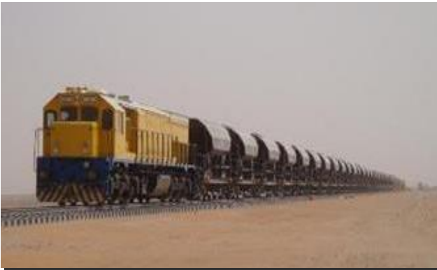
THE NORTH-SOUTH RAILWAY PROJECT CIVIL & TRACK WORKS, RAS AS ZAWR TO AZ JABIRA
