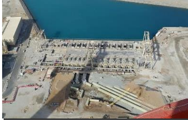
JEDDAH SOUTH THERMAL POWER PLANT (4x700 MW), STAGE 1
